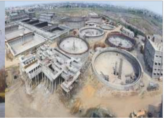
130 mld STP to reuse water for TPS Koradi
