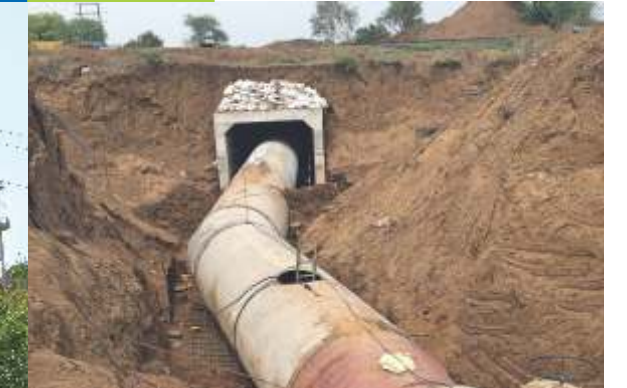
2300mm MS Pipe Line Railway Crossing
