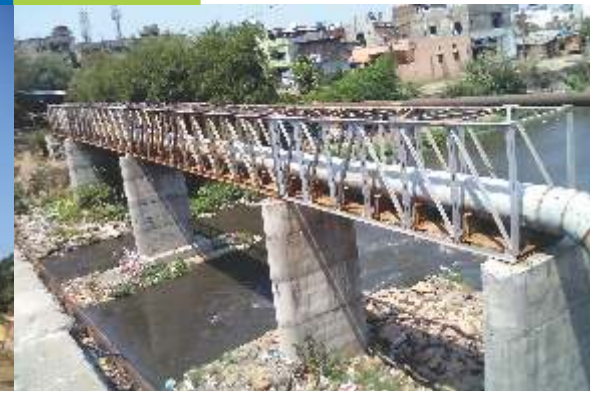
Pardi Bridge Feeder Main
