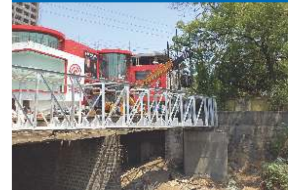
Bridge for Feedermain
