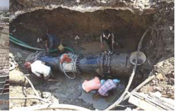
Installation for Flow Meter
